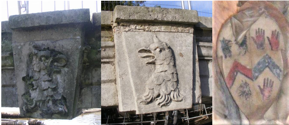
Fig 6 and 7 (left and centre); The north and south facing keystones. Note the thick band of mortar between the top of each stone and the coping above. Fig 8 (right) – The Scawen arms impaled with those of the family of Dame Mary Scawen nee Maynard, from her monument in All Saints Parish Church, Carshalton, c.1700.
