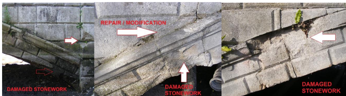
Examples of damage to the elevations - Fig 13 (left) North elevation, west side; figs 14 and 15 (centre and right) South elevation, west side.
