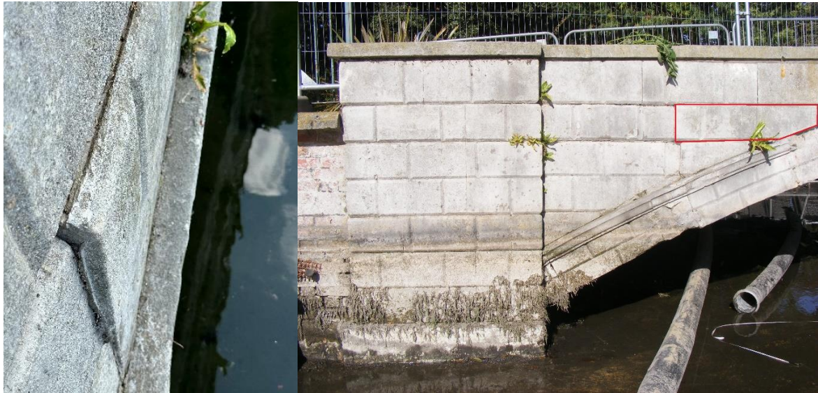
Figs 11 and 12 – spalled stone panels on the north and south elevations
