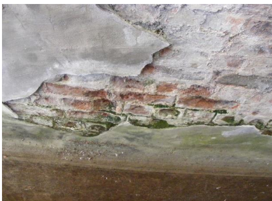
Fig 10 – the vault soffit, showing the degraded concrete scree and brickwork.
