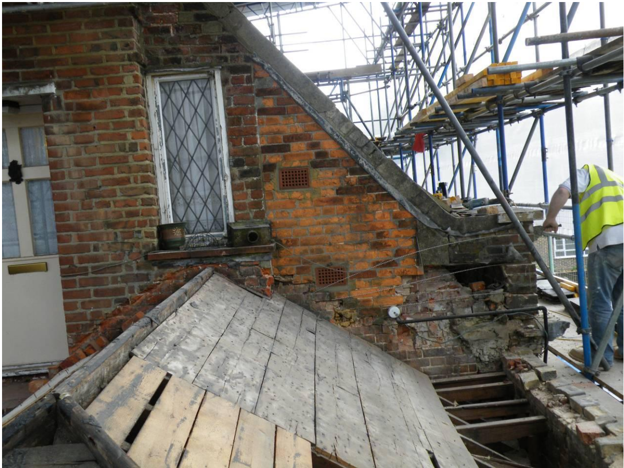
Figure 9. The western (front) end of the north gable of the main block. Note the bonding break and mathematical tiles to the right.
